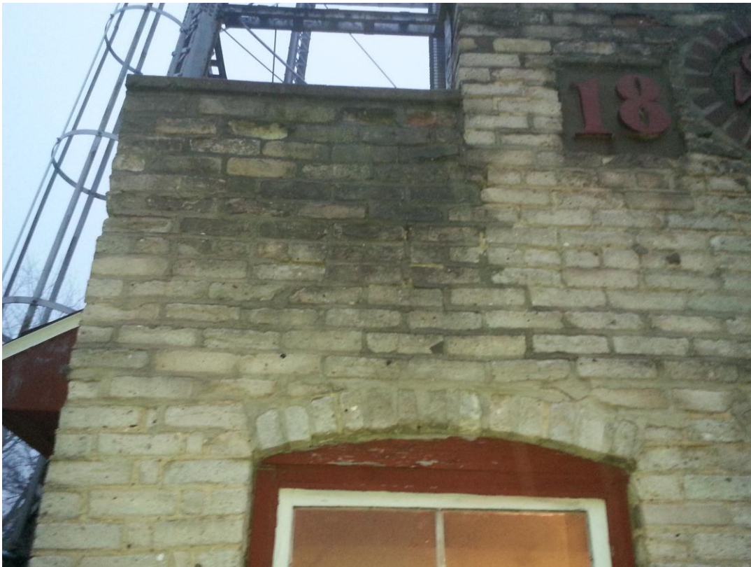
Brick needs to be repointed and cleaned.
